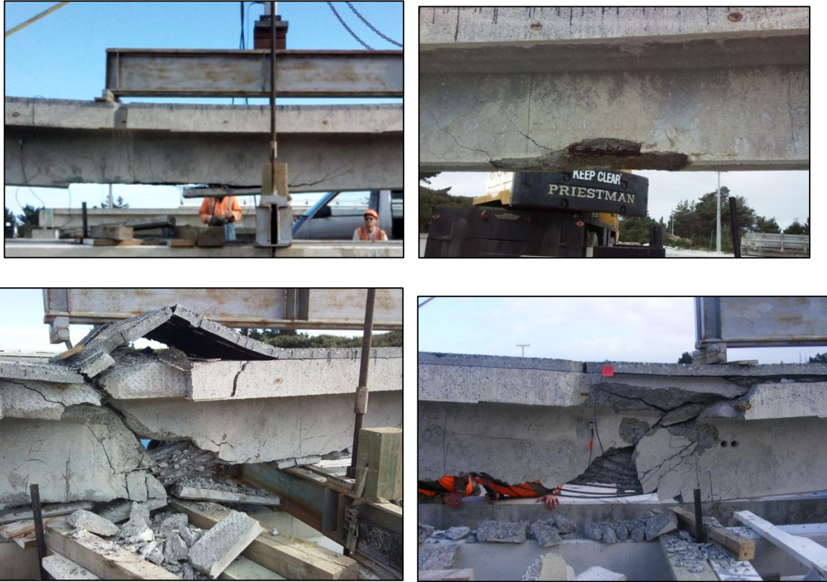
Fig. 11 Typical corroded beam cracking and failure
