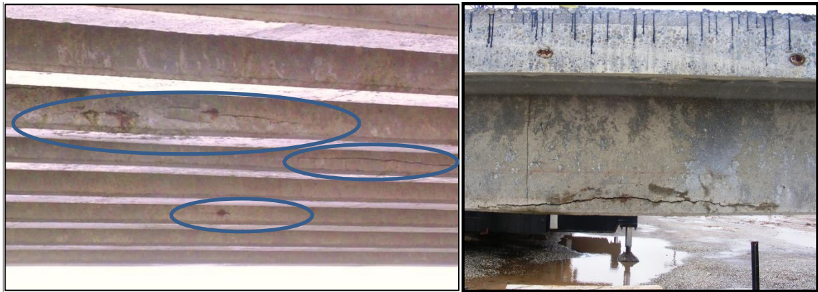
Fig. 2 Corrosion induced cracking in side of web near soffit
