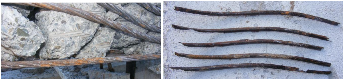
Fig. 5 Strands with uniform corrosion and individual wires with pitting damage
