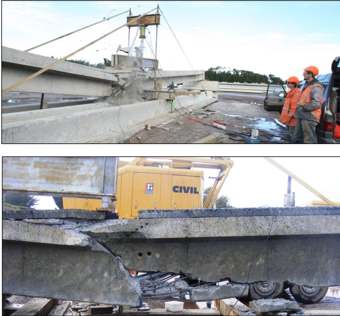
Fig. 10: Typical good condition beam failures
