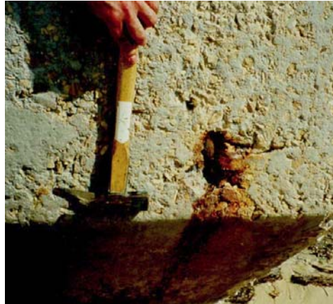
Figure 6: Corrosion of bridge in Progresso containing stainless steel reinforcing.
