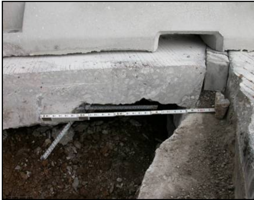
Figure 1. Deteriorated paving notch on an integral abutment bridge.
