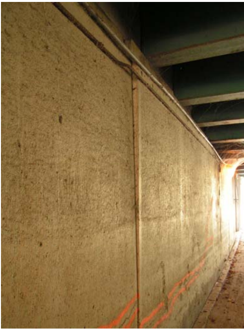
Fig. 4 – Differential Wall Movement
