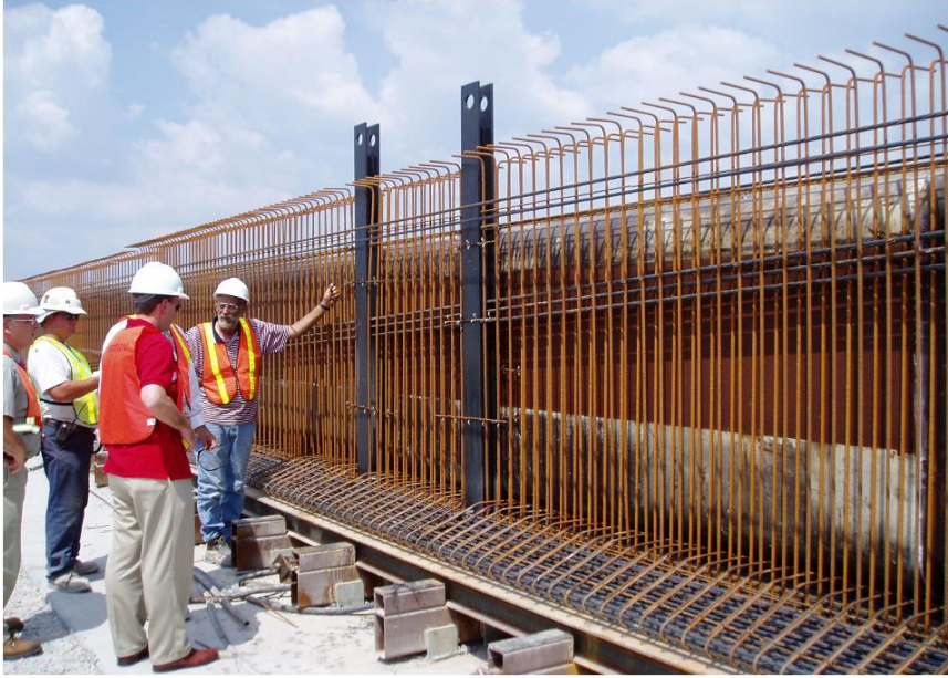
Fig.2- Stiff plate inserts at 14 ft from the ends of a 175-ft, 6-ft-deep girder, with lift holes high above tops of reinforcement. The girders should be stored in the precast yard on rigid dunnage in a north-south direction to avoid bowing due to uneven exposure to the sun.
