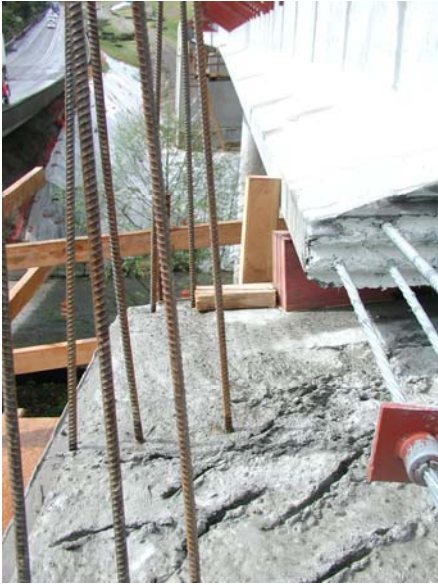
Fig. 6- Precast girder set on oak blocking before the entire girder end is enclosed in a concrete cross beam.
