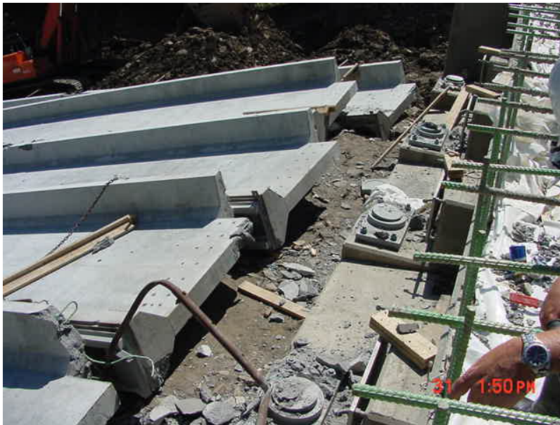
Fig. 1- Collapsed precast concrete girders that had been placed on circular pot bearings with Teflon and a narrow stainless steel sliding assembly.
