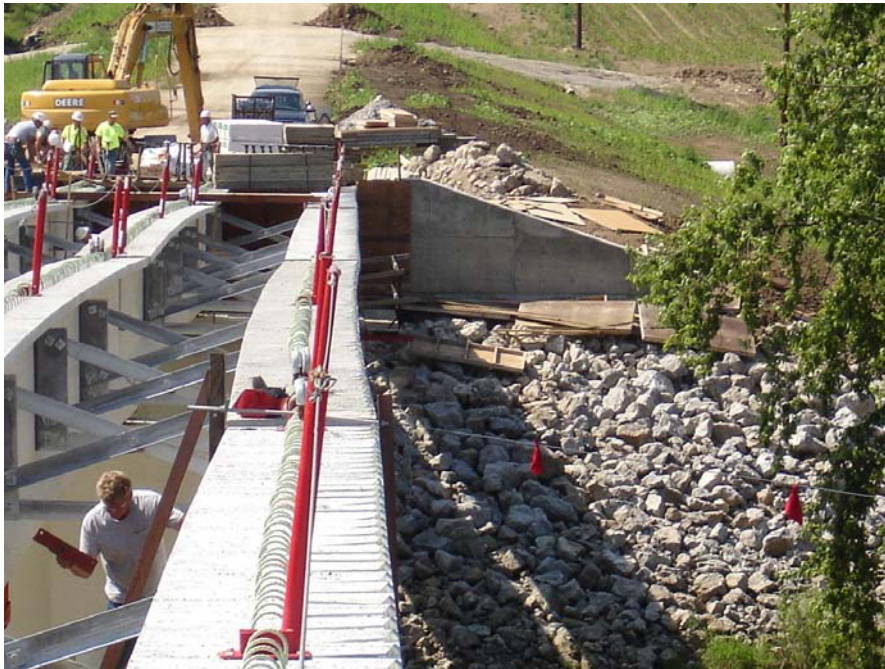
Figure 8- Lateral deformation subsequently removed by plumbing beam ends and reattaching cross bracing to the straightened girder.
