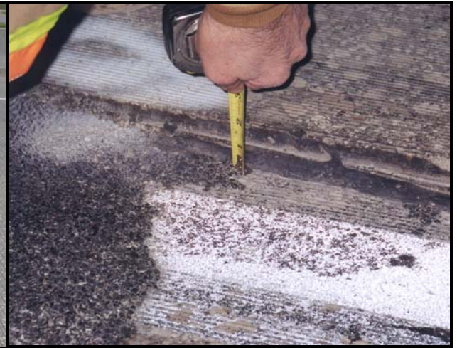
Fig. 2 Approach pavement settlement
