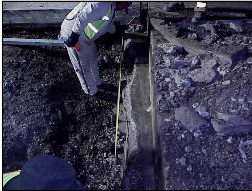
Fig. 11 Deteriorated paving notch on an integral abutment bridge.
