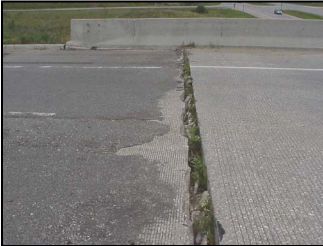
Fig. 1 “The bump at the end of the bridge”
