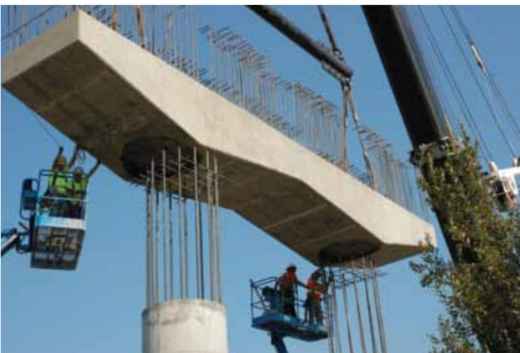
Figure 4. Previous use of precast concrete cap beam that used a large number of column bars in a seismic area of Washington State.
