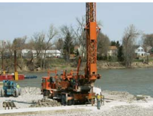
As one requirement of construction was to not disturb the fish spawning grounds in the river, shafts were drilled through the existing piers to avoid any disruption. To facilitate drilling through the old piers, they were cut off at the water line during demolition, and a leveling course was cast before drilling the new shafts.
