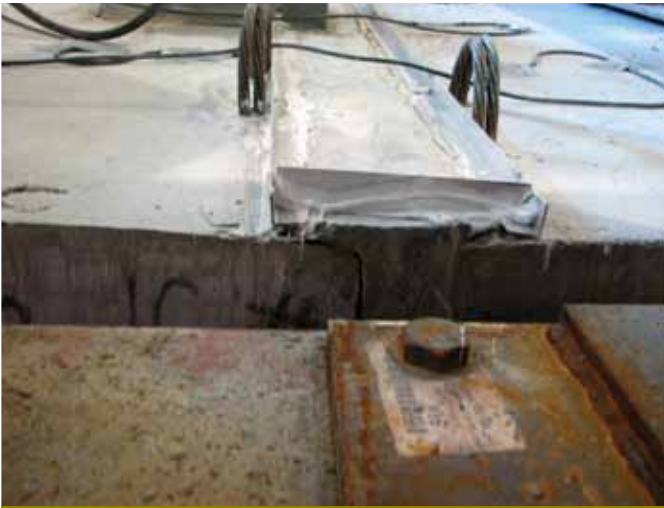
Figure 10. Failure of the current connection without topping.
