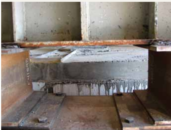
Figure 11. Failure of the current system.
