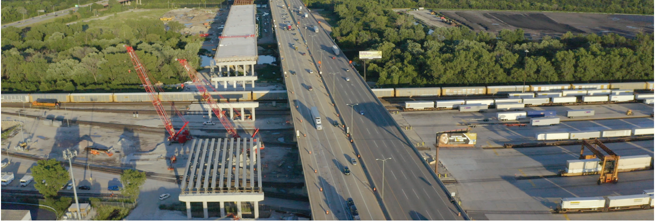
County Prestress & Precast LLC of Janesville, Wis., (formerly operating as County Materials Corp. at the time of this project) manufactured and delivered 523 prestressed concrete girders for the Mile-Long Bridge in Chicago, Ill. Courtesy of County Materials Corp.
