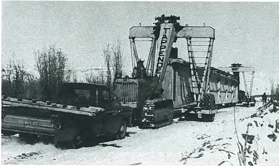
Fig. 27. Handling the 148-ft (45.1 m) post-tensioned girders for the Duchess Bridge on Highway 36 across the Red Deer River.
