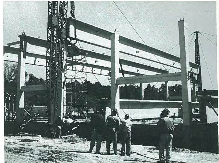
Fig. 40. Girder No. 3 almost in position over columns. The column cables are being pulled up in order to thread them through holes in the girder ends.
