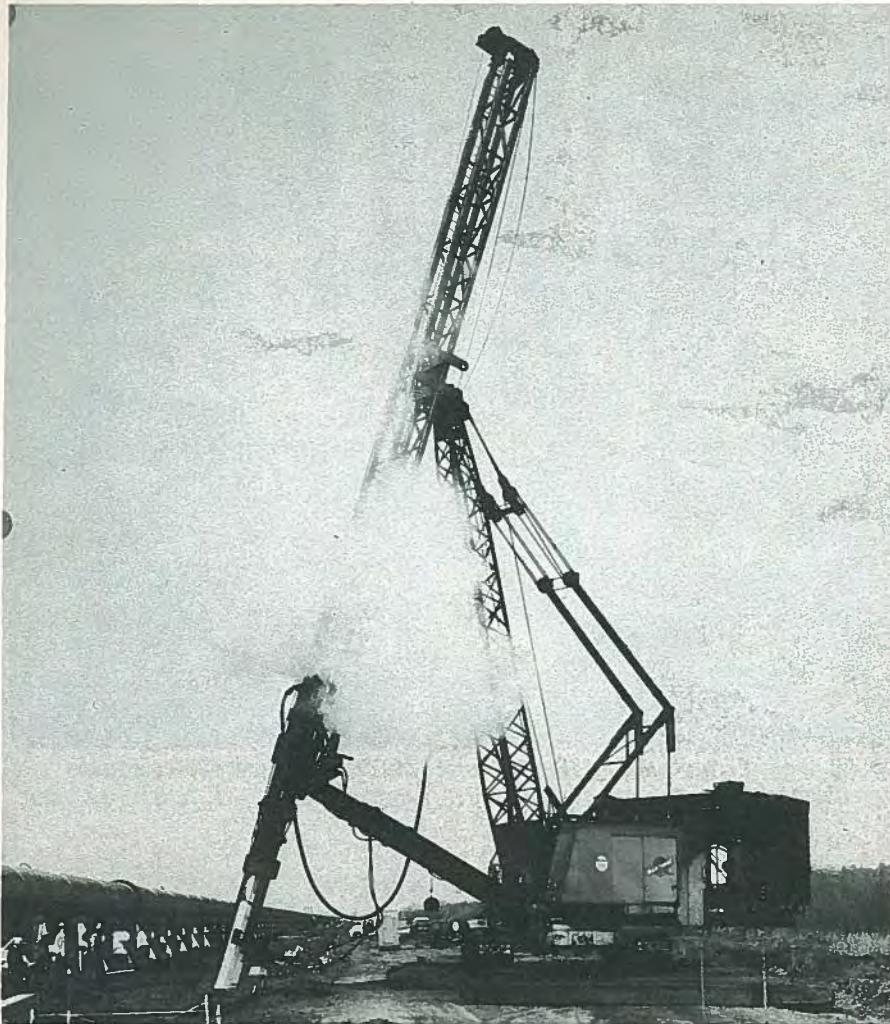
Fig. 51. East of San Francisco, 1966: driving of 5000 pretensioned concrete piles, all on a batter, to support 72 in. diameter steel water pipe across 10 miles of marshland.
