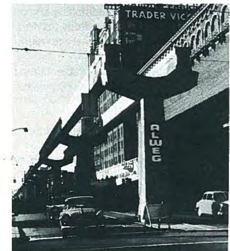
Fig. 88 View of the Seattle Monorail under construction, showing the cross section of the girders, and the shape of the support columns, on a straight stretch of the beamway.
